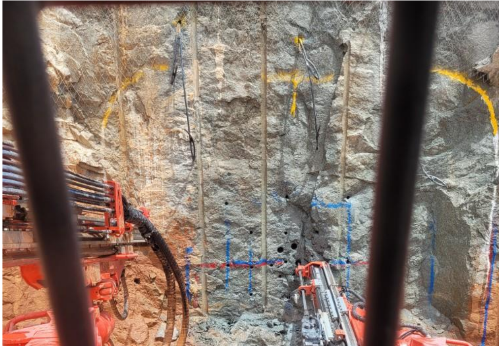
View from inside the new Sandvik Twin Boom Jumbo preparing the Cassini portal for first firing
